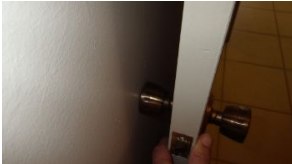
few door stops were present. Damage may result from knobs hitting the drywall.
