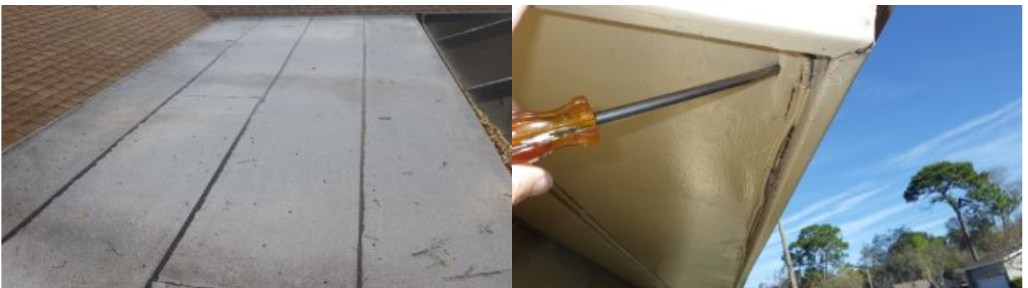
The flat roof over the rear patio appears to be the same age.
