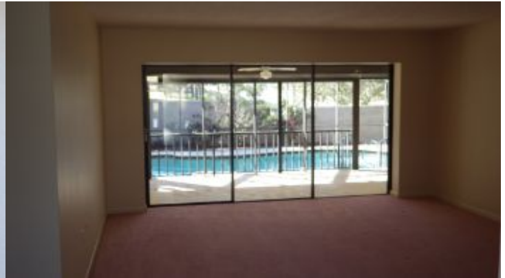
Patio doors are operational. Continue normal maintenance such as cleaning and lubricating
