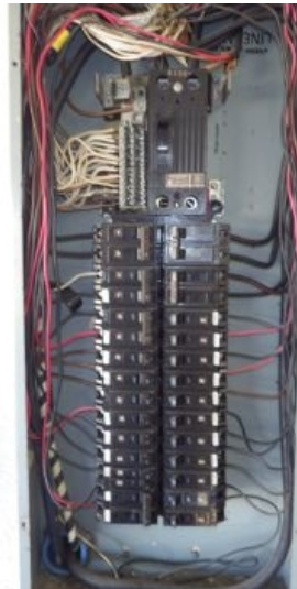
Removal of the cover panel on the circuit breaker panel revealed no significant issues, except as noted.
