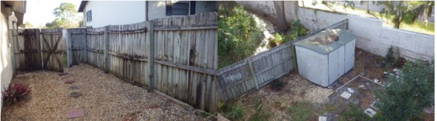
Wooden privacy fence is in poor condition with some missing slats, staining and panels not entirely secured to posts.
