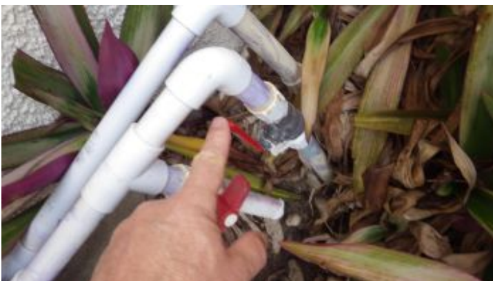
The main water shutoff valve is located on the east side of the house at the water conditioner.
