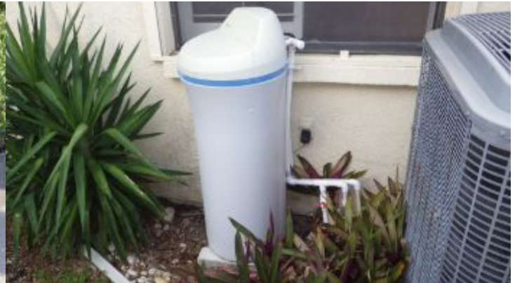
A water conditioner system is present in the house (on the east side outdoors) and Does appear to be functional.
