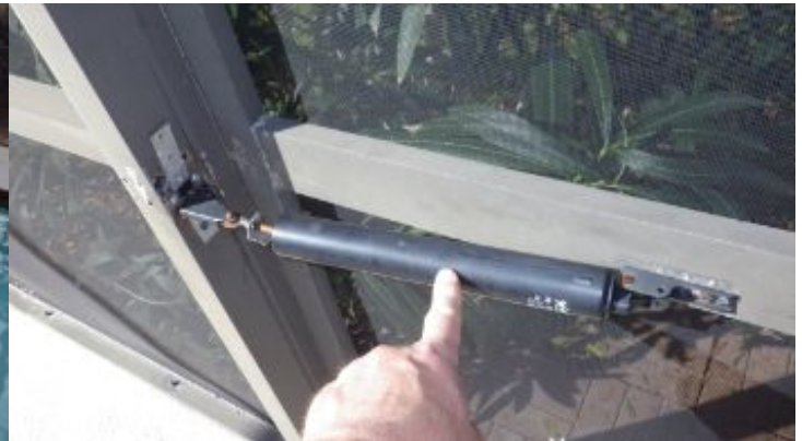
Both screen doors have issues with latches and piston closers.
