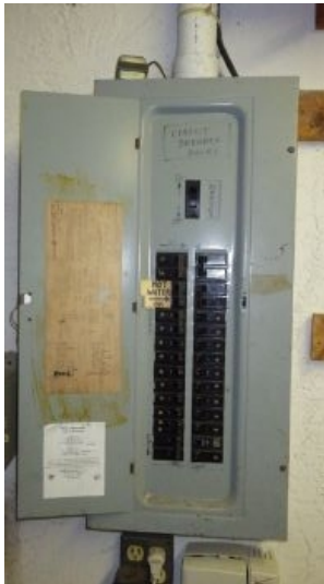
The main breaker panel is located in the garage.
