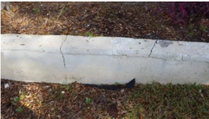
masonry retaining wall near fireplace is cracking in several spots.
