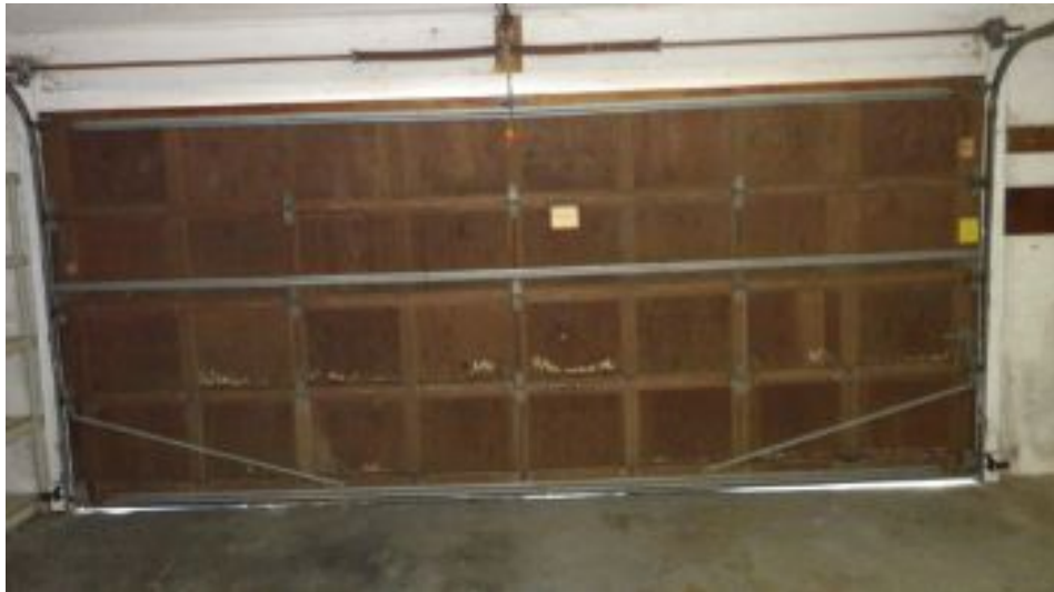
One original 16' wooden door with torsion lift spring. Minor wood stains from various leaks but door appears intact.
