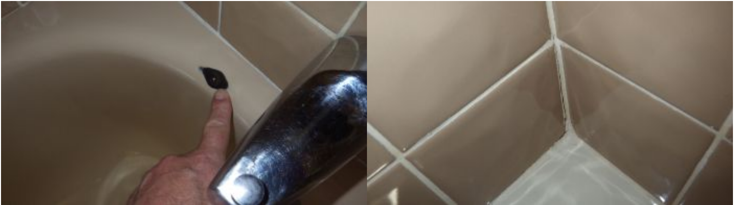
There was a large chip observed in the tub in the hall bath
