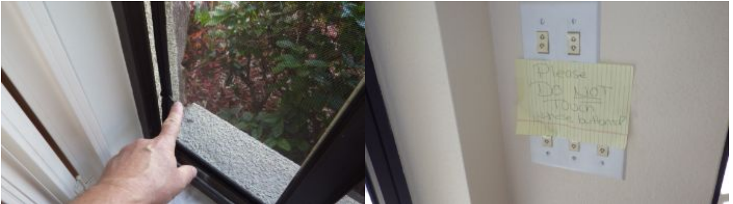
Screens are damaged or frayed in a few windows.
