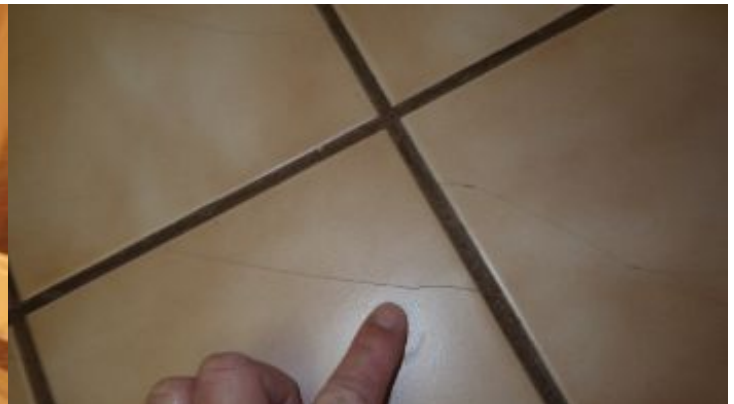
The tile floor in the hall bath is not secure to the substrate. The tiles are cracking, because they do not stick to the subfloor.
