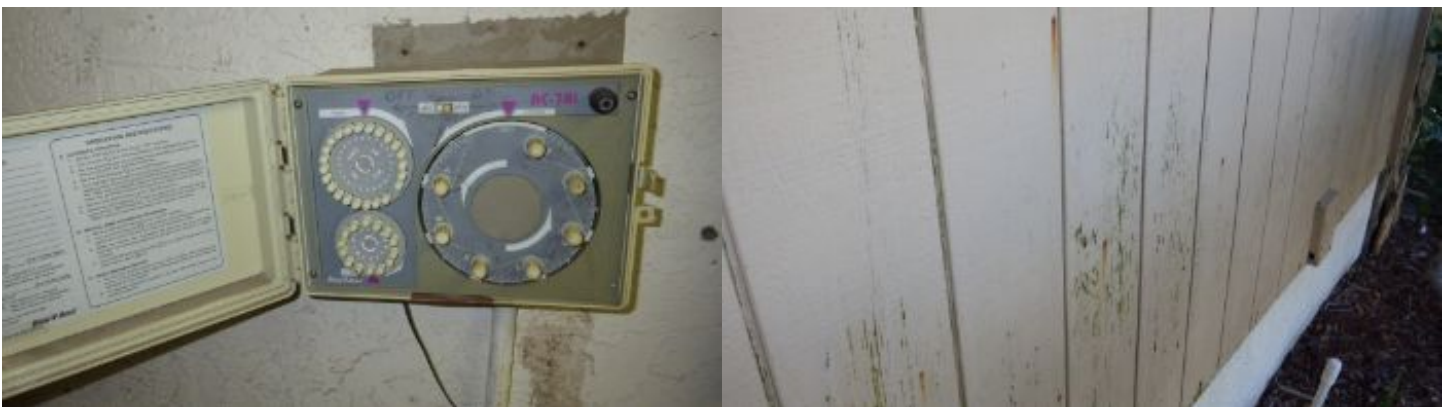
A 7 Zone irrigation system was present and operated normally.
