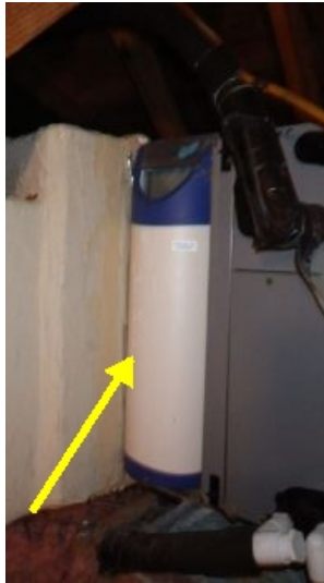
System filter sizes: (large pleated type in the main return air line in the attic)
