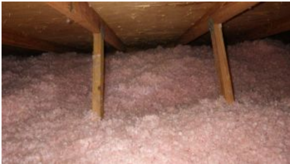
Blown in fiberglass on top of the old style rockwool fiberglass was observed in the attic.
