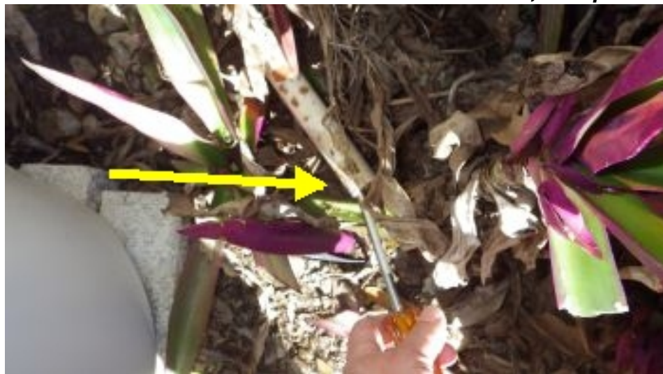
Condensate drain line is buried in plants behind the compressor.
