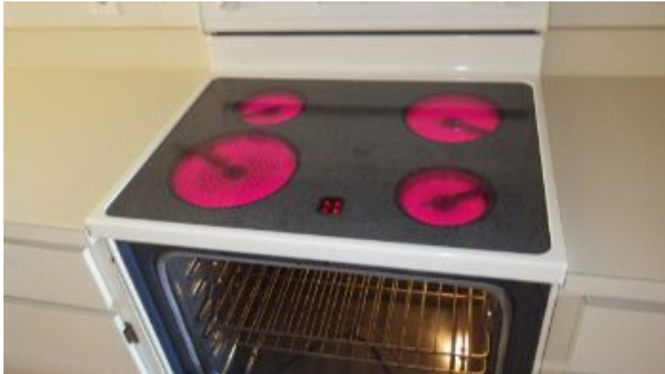
All heating elements operated when tested.
