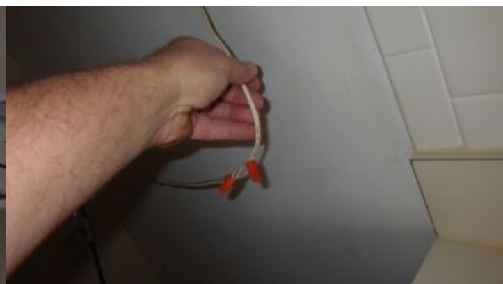
Under counter fluorescent lighting is using a spliced, wire nutted, lamp cord for power source. See behind the refrigerator.
