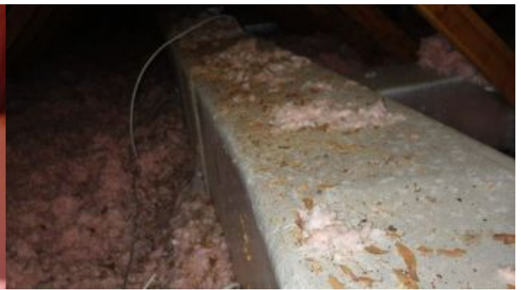
Duct work was primarily located in the attic, and appeared to be in satisfactory condition overall, except as noted.
