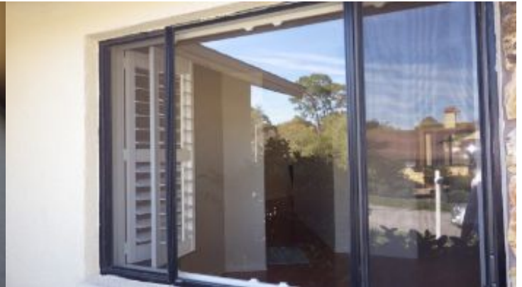
All tested windows were operational, except as noted Most are single hung single glazed, non impact windows with a few sliders.
