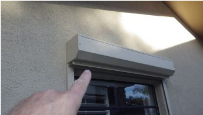
All roll down storm panels appeared operational except the one on the west side of the patio.
