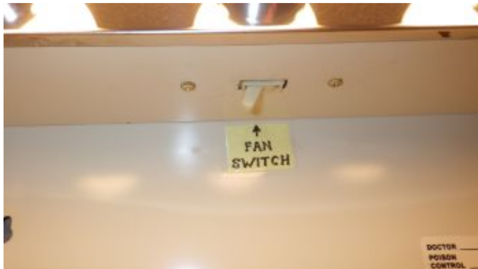
Non Standard workmanship for a light fixture and switch for the exhaust fan in the half bath.
