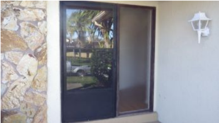
No major issues noted with any doors. All appeared operational and intact, except as noted.
