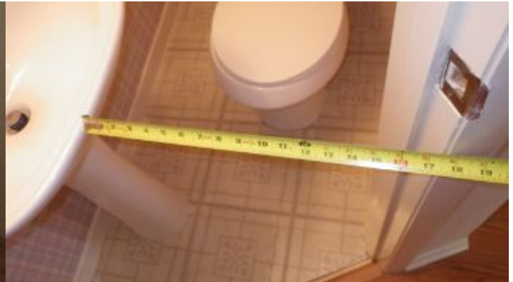
Non standard construction of the half bath. The room appears to be a modified closet.
