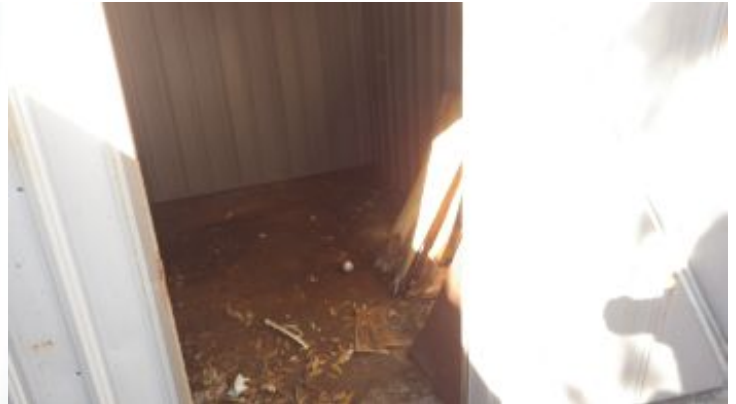
The metal shed doors were rusty, and the wood deck appears to be decayed and stained.
