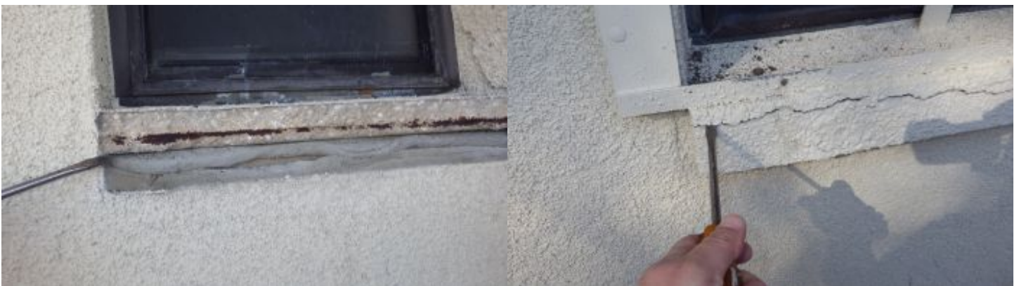
Window sills are made of concrete and several were noted as damaged or cracking. The one on the master bath window (West side) was broken right off
