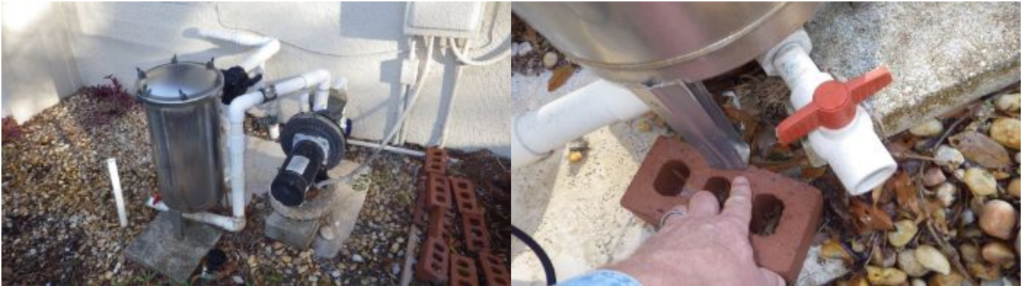
A single pump, no chlorinator, no flow control valves, and a stainless steel cartridge filter housing all appear to be fully operational.
