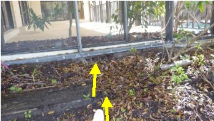
Wooden retaining wall on west side is severely decayed and a large section has failed. The garden above the retaining wall has washed away with the deck of the patio losing support.
