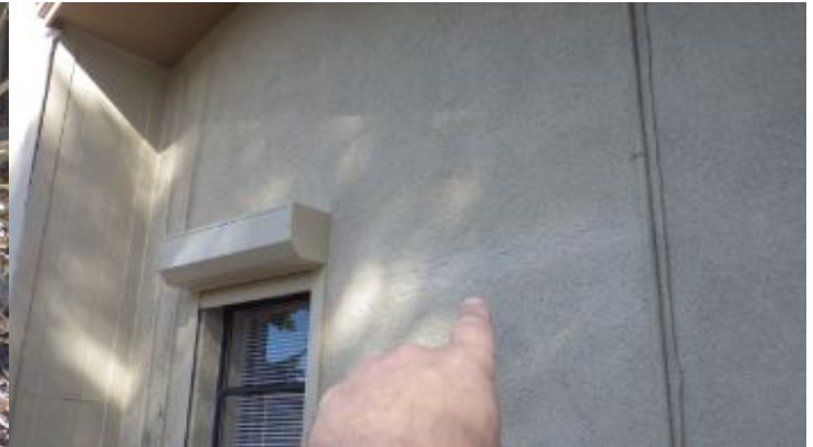
Obvious crack covered by stucco spray texture.
