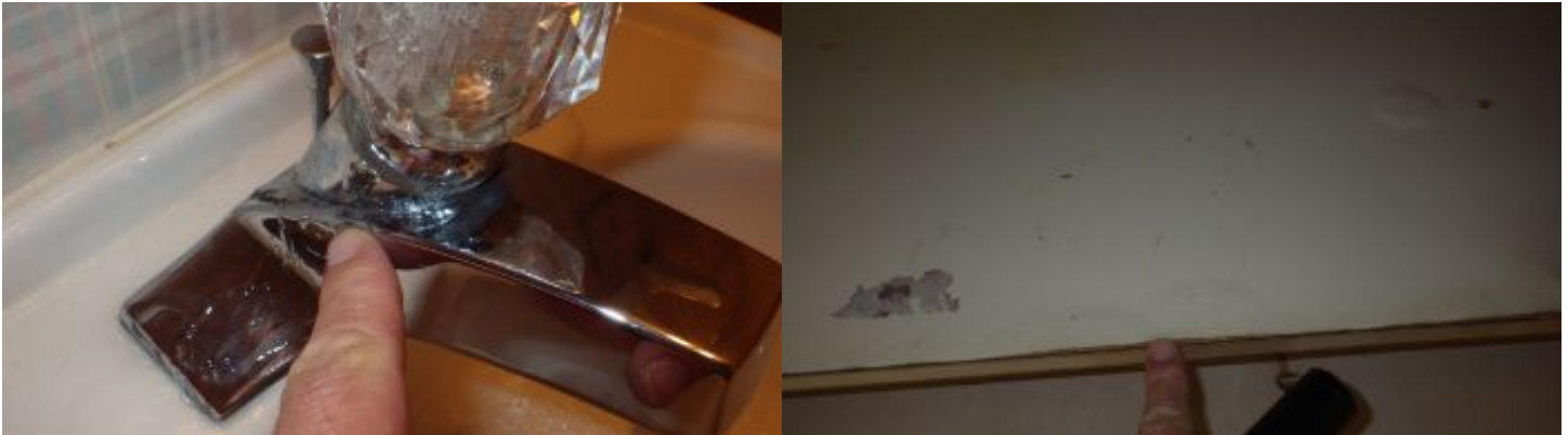
Faucet leaks at handle in half bath when in use on cold.
