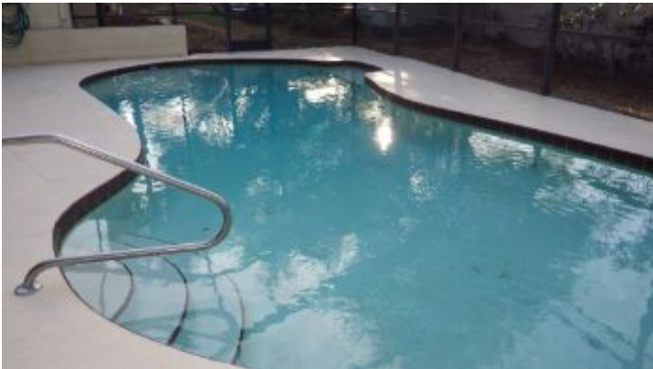
Pool plaster finish has served its useful life and is damaged. The concrete is showing through the plaster in some spots.
