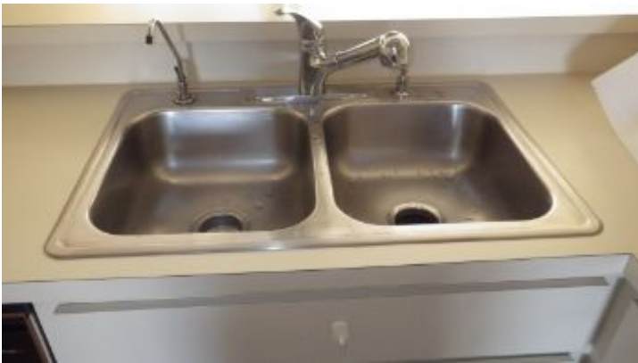
Kitchen has a Stainless steel - surface mounted sink
