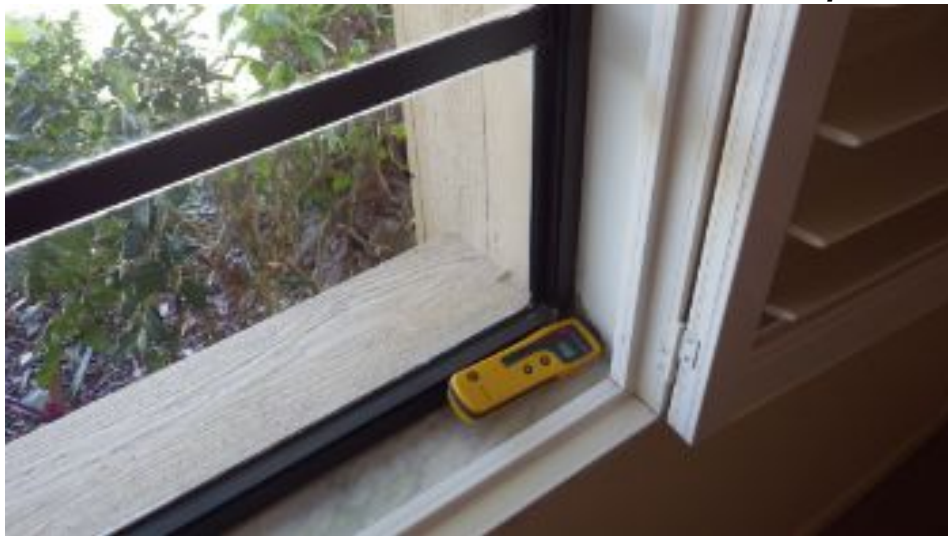
High moisture readings noted at the windows in several rooms
