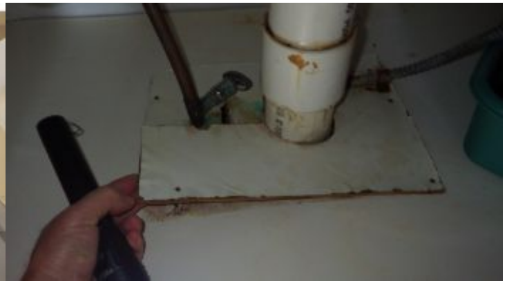
The sink cabinet base wood was slightly damaged by presumed past leaking.
