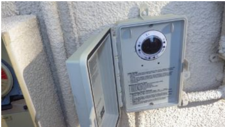
Sub-panel with timer control for pump present. The mechanical timer in the sub-panel was abandoned for a programmable timer in an adjacent box.
